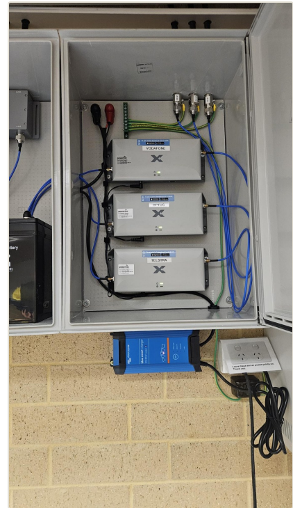
One Cel-Fi unit per carrier — Telstra, Optus and Vodafone — inside a single equipment cabinet.
