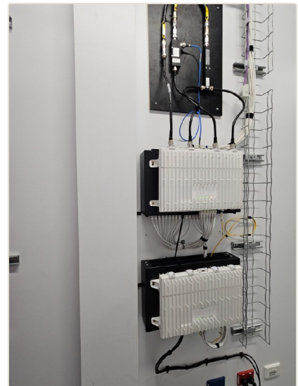
Cel-Fi Quatra network units, wall-mounted as part of an equipment cabinet.
